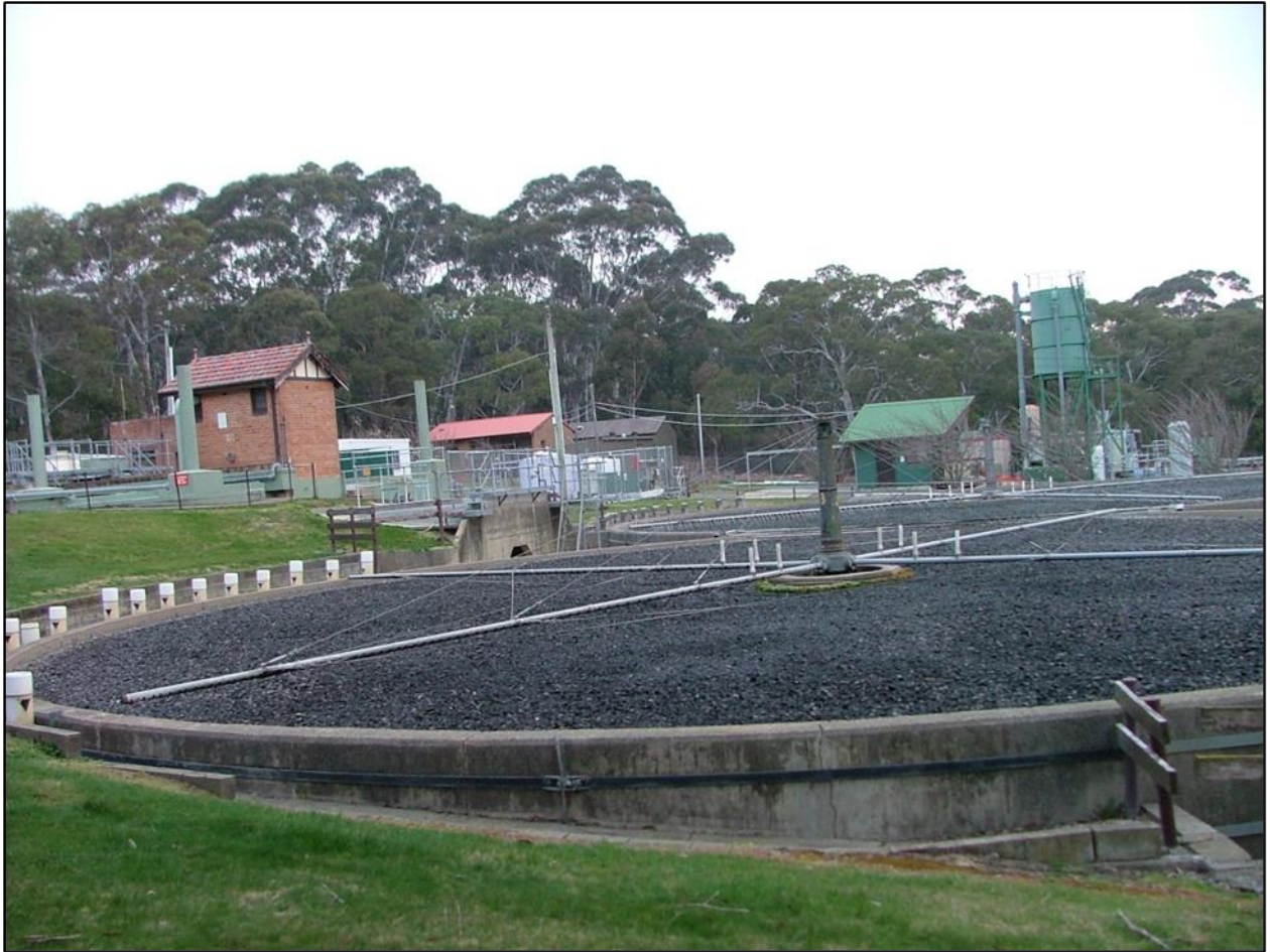
Figure 19. Aged trickling filter technology at the Blackheath sewage treatment that closed in 2009. Photo Ian Wright.
